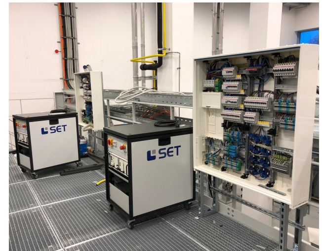
Power Grid Control
